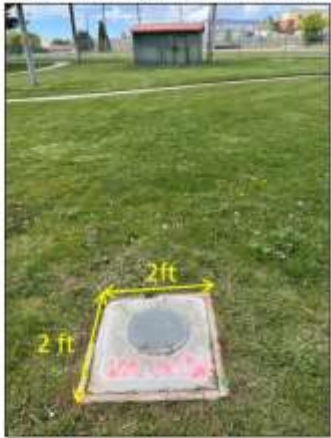
Monitoring Well in Park
