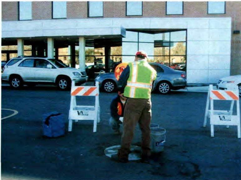
East Side Springs View: South 11/16/11 EPA-MW-05. Bailing EPA monitoring well EPA-MW-05 located in the Veteran's Affairs Hospital parking area north of Building 16.
