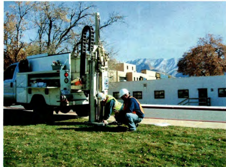
East Side Springs View: Southeast 11/16/11 URS leak testing at soil-gas location ESS-SG-30. Sample located in the southeast corner of grassy area south of Building 16.
