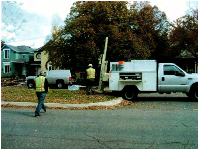
East Side Springs View: East 11/15/11 URS setting up the direct-push unit at ESS-GW-11 (818 South 600 East ).
