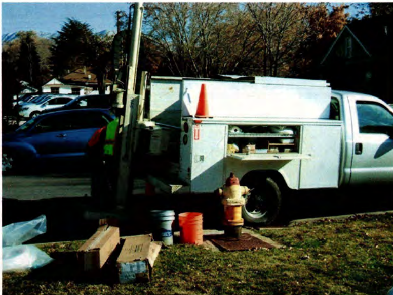
East Side Springs View: East 11/14/11 URS setting up the direct-push unit at 920 South Lincoln. DERR abandoned the location after meeting refusal at 24 feet bgs.
