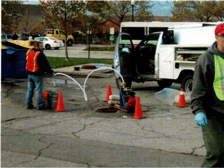
East Side Springs View: Southwest 11/14/11 URS setting up the inertia pump at EPA-MW-01S. The well is located in southwest corner of SLC Sports Complex parking area. (Photo: MWH)
