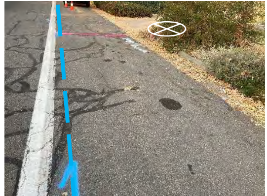
Water line located running up the street adjacent to planter where GW-20 was located in the planter area.
