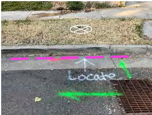
Storm water lines and unknown line located in street adjacent form existing GW-16 location
