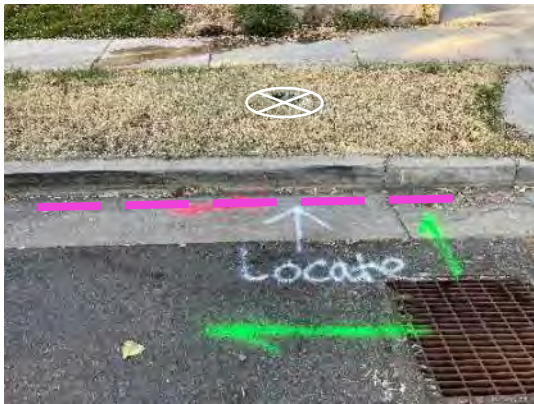
Storm water lines and unknown line located in street adjacent form existing GW-16 location
