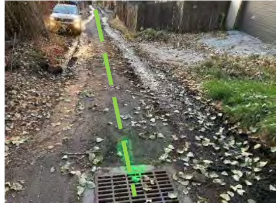
GW-11, storm water drainage runs down the alley approximately in the middle of the road.
