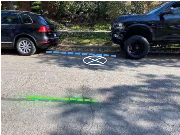
MW 38 (Elizabeth Street option) note proximity of water line markings. Sewer in center of street, recommend engaging Blue Stake before proceeding.
